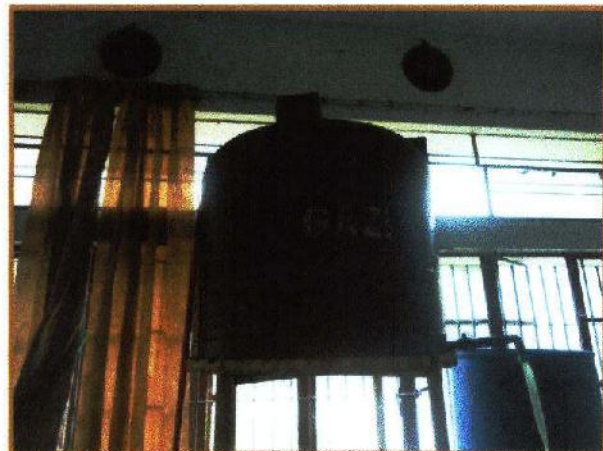
Fig-8: Overhead Tank
